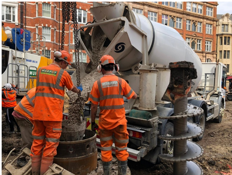
AACM Concrete used for piling contract in London (Courtesy of DB Group)
